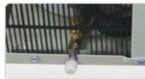
Cold tank drain
