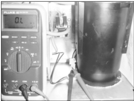
Picture 18. Blower Open Motor
