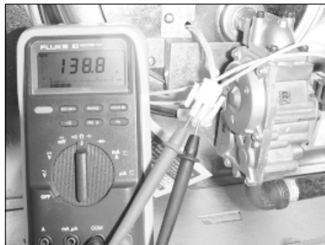
Picture 22. Test Hot Surface Ignitor
