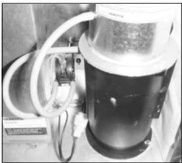
Picture 15. Combustion Air Blower
