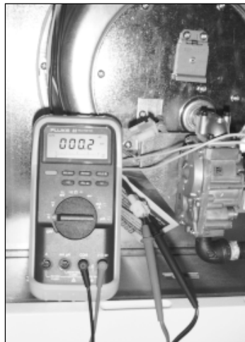
Picture 21. Ignitor and Voltmeter
