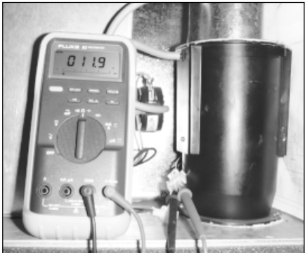
Picture 17. Blower OHM
