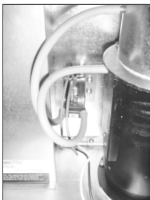
Picture 19. Pressure Switch
