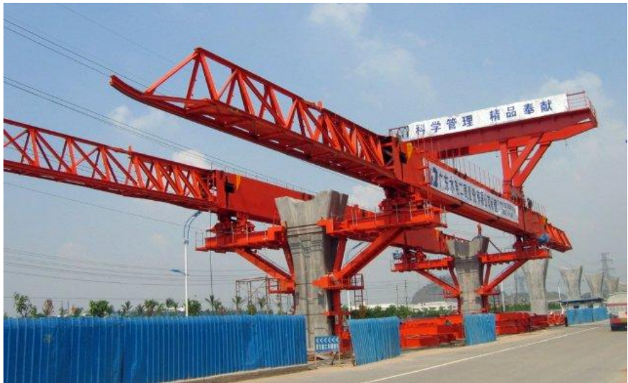
Figure 12: 76m, 325ton underslung gantry with 40ton crane for 35m, 490ton dual-track LRT spans (NRS)
