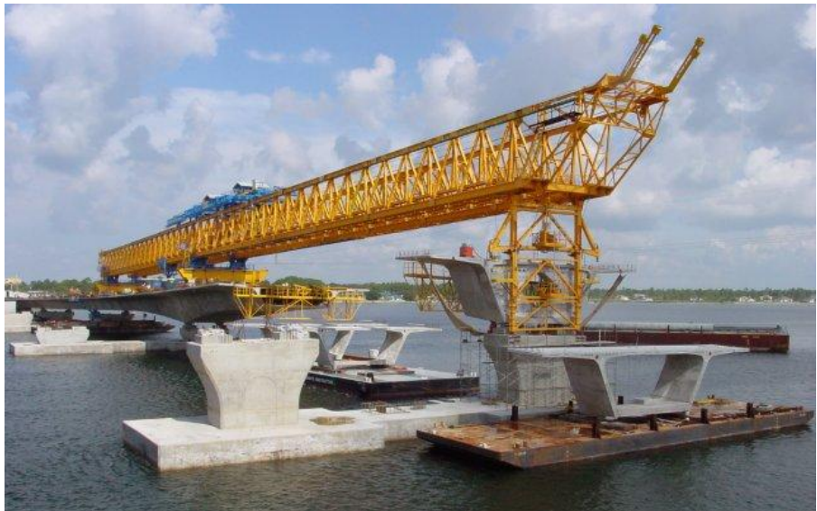
Figure 27: Placement of the first 182ton down-station segment with a 198m, 876ton gantry for 101m spans (HNTB)
