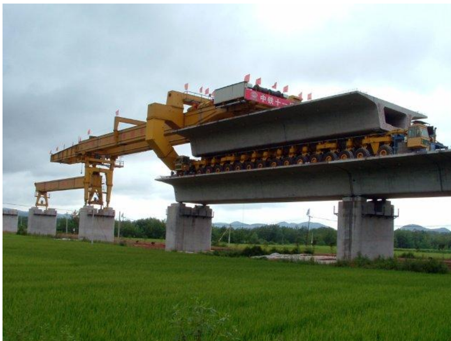
Figure 36: 75m, 520ton gantry with 38m, 80ton underbridge for placement of 33m, 900ton dual-track HSR spans (Beijing Wowjoint Machinery)
