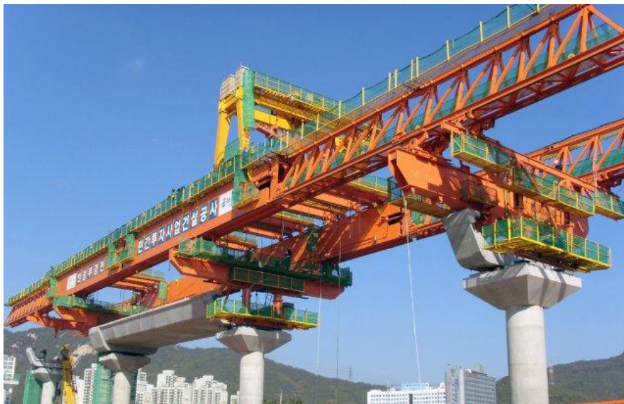
Figure 3: 98m, 405ton overhead gantry with 45ton portal crane for 45m, 500ton dual-track U-girder LRT spans (NRS)
