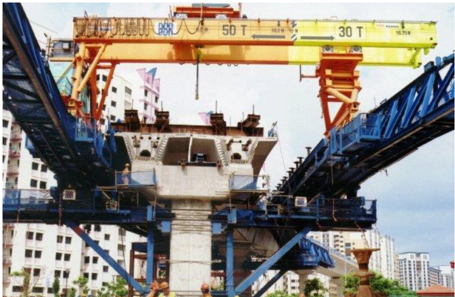
Figure 13: 91m, 333ton pivoted underslung gantry with 40ton crane for 36.7m, 392ton dual-track LRT spans (NRS)
