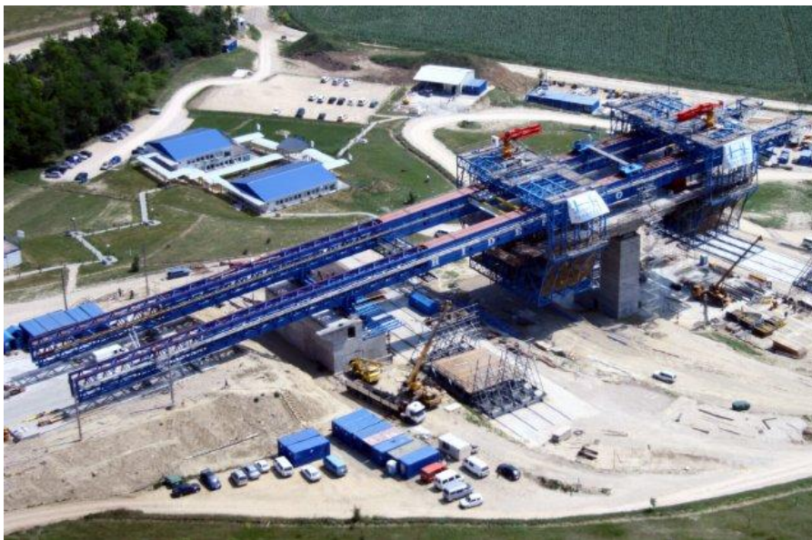
Figure 32: 158m, 1600ton MSS for balanced cantilever casting of 120m spans with 11.3m, 680ton two-phase segments (ThyssenKrupp)
