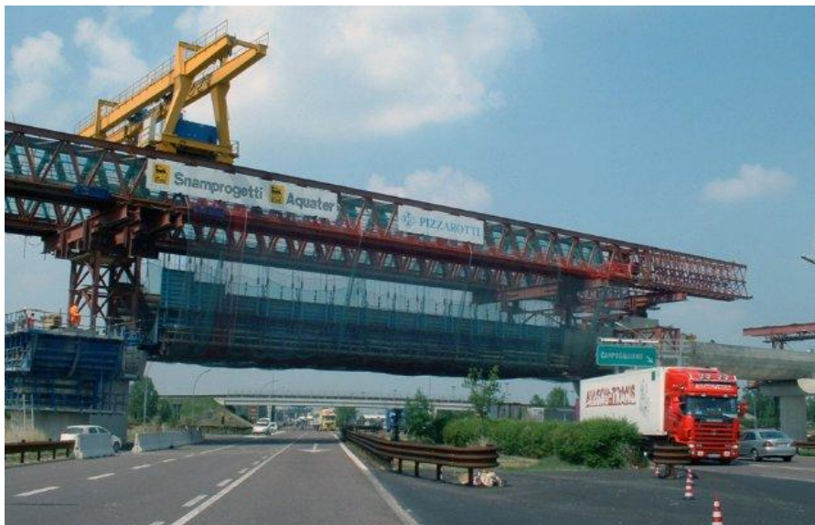
Figure 15: 110m, 1490ton overhead MSS with 60ton crane for 57.4m, 1380ton single-track HSR spans
