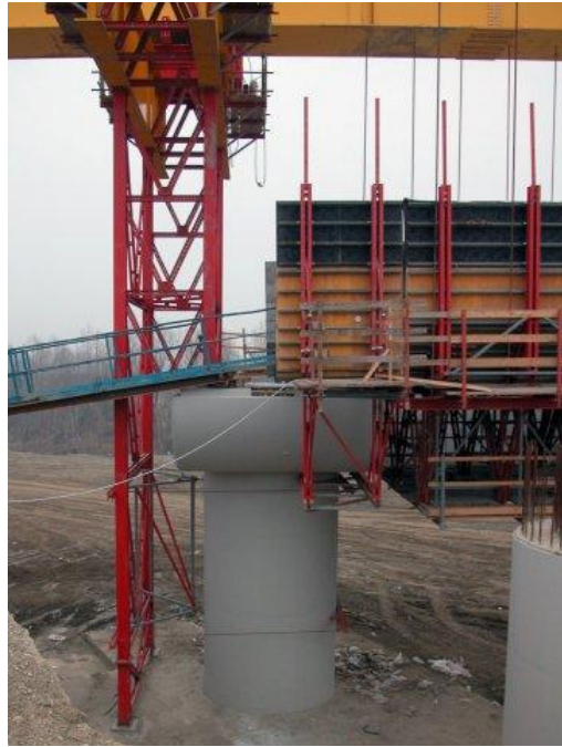
Figure 42: Bracing deficiencies in a 19m support tower
