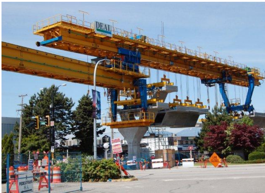
Figure 11: 41m, 96ton underbridge and 47m, 132ton main girder for 37m, 340ton dual-track LRT spans (Deal)
