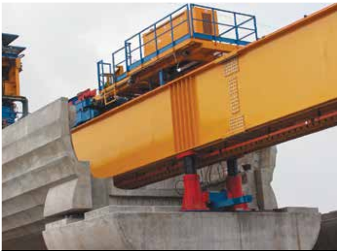
Figure 15. Motorized saddle on the rear overhang of the underbridge.
