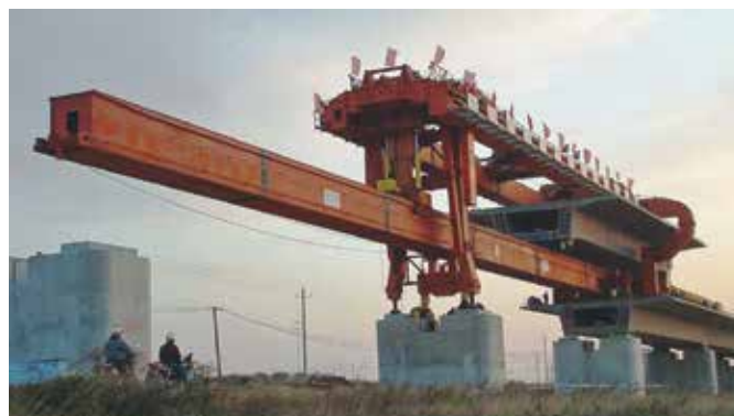
Figure 12. Short launcher with two-span underbridge for 32.7 m (107 ft), 9000 kN (2020 kip) dual-track box girders. Courtesy of BWM.
