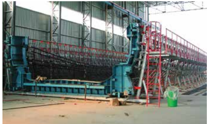
Figure 4. Reinforcing bar jig for full-span cage prefabrication of a single-track U beam.
