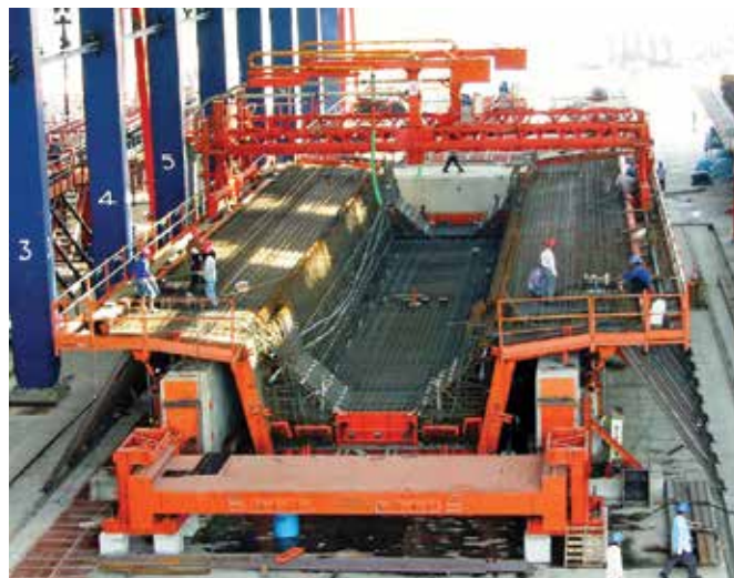
Figure 6. Casting cell for combined pre- and posttensioning. Courtesy of VSL.
