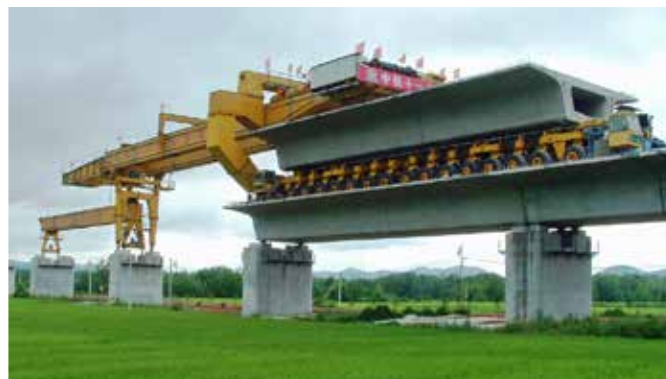
Figure 11. Telescopic beam launcher for 32.7 m (107 ft), 9000 kN (2020 kip) dual-track box girders. Courtesy of BWM.
