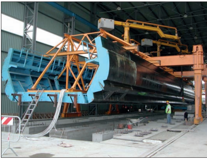
Fig. 3: Rail-mounted inner form
