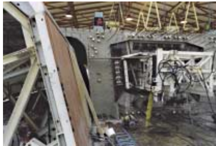
Fig. 3: Rear end of the self-extracting internal form for the bridge of Fig. 4 (author).
