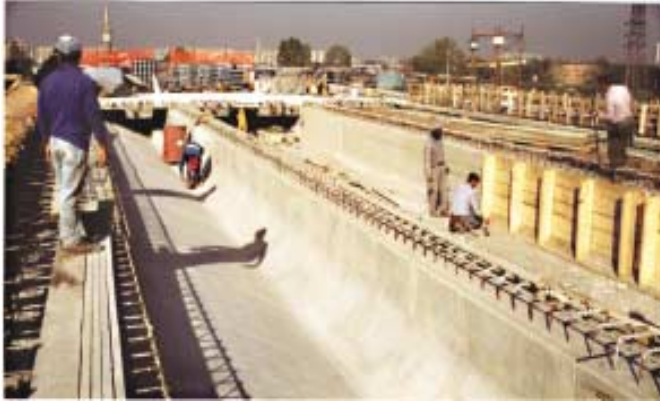
Fig. 11: Construction joints at the top slab level ease dismantling of internal form and removal of rubble (author).
