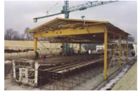
Fig. 2: Preassembled cage of a 24.0 m (80 ft.) segment with precast anchor blocks. On the right, the main formwork (author).
