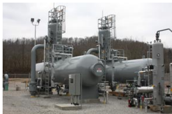
Completed pressure vessel system which cleans the natural gas after it is extracted out of deep underground wells.
