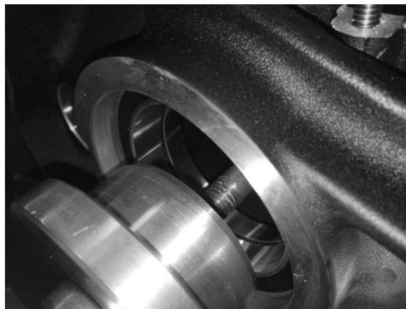
FIGURE 17 | TAPERED BEARING ADAPTER VISUAL INSPECTION
