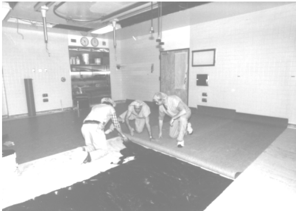
Fig. 3.4.2.2 Folding Back Vinyl and Troweling Approx. 200 sft. (shown with a black Conductive Adhesive not UZIN KE 2000 SL conductive adhesive)
