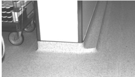
Fig. 3.6.1 Example of Three-Dimensional Coving. With Hot air Putty Technologies, as Described Under Flash Coved Corners.
