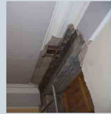
No Job Too Small: This is a very typical day's work within our company, reinstating a section of plain moulded cornice – in this particular instance, cut out above a doorway during renovation works.
