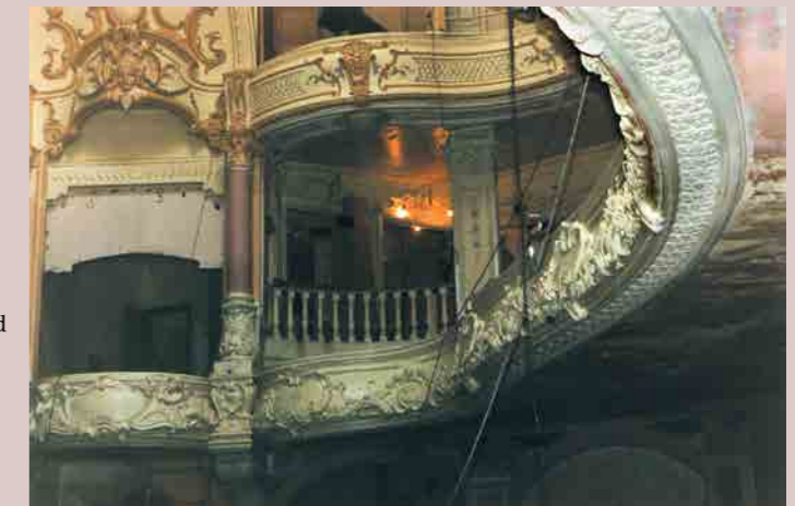
Glasgow's Pavilion Theatre: Pictured above is the reinstatement of curved ornate plaster mouldings to the underside of the balcony.
