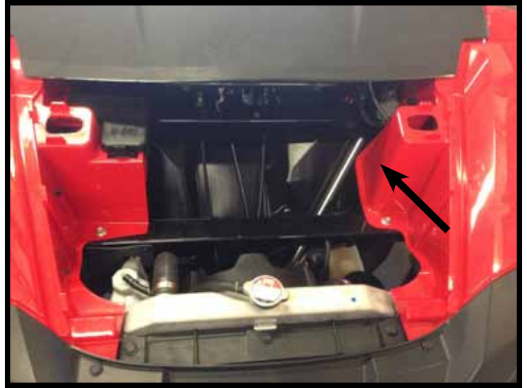
“Figure 7” Contactor Location
