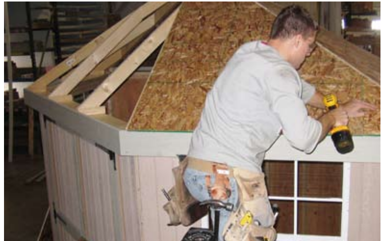
42. Locate sheathing that goes on top of rafters. Fasten sheathing with 1 1/4" screws every 8" on center.
