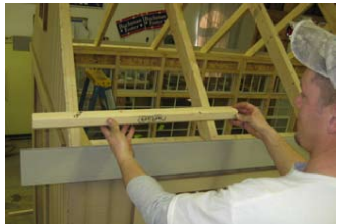
54. Purlins will be installed on top of trusses for Sunsky to set on.
