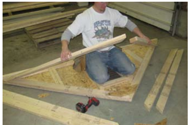
42. Next locate gable wall and use it for truss assemble as shown.
