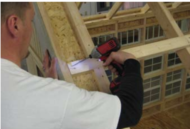
77. Continue with 2 1/2" screw going from top of purlin into the rake on an angle.
