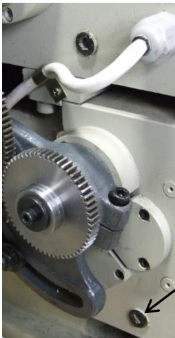
Gearbox Oil Drain
