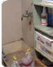
Cleaning Chemical Storage (Janitor's Closets)
