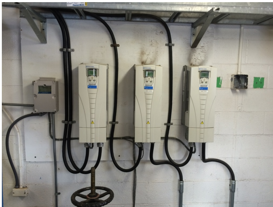
Variable Frequency Drives for Submersible Distribution Pumps
