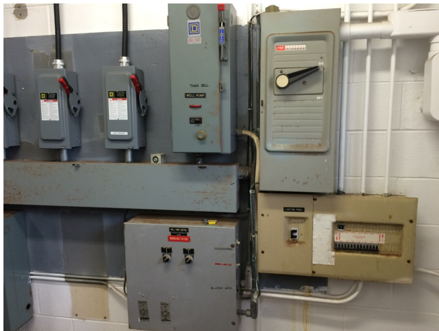
Right Side of Electrical Panel Cluster
