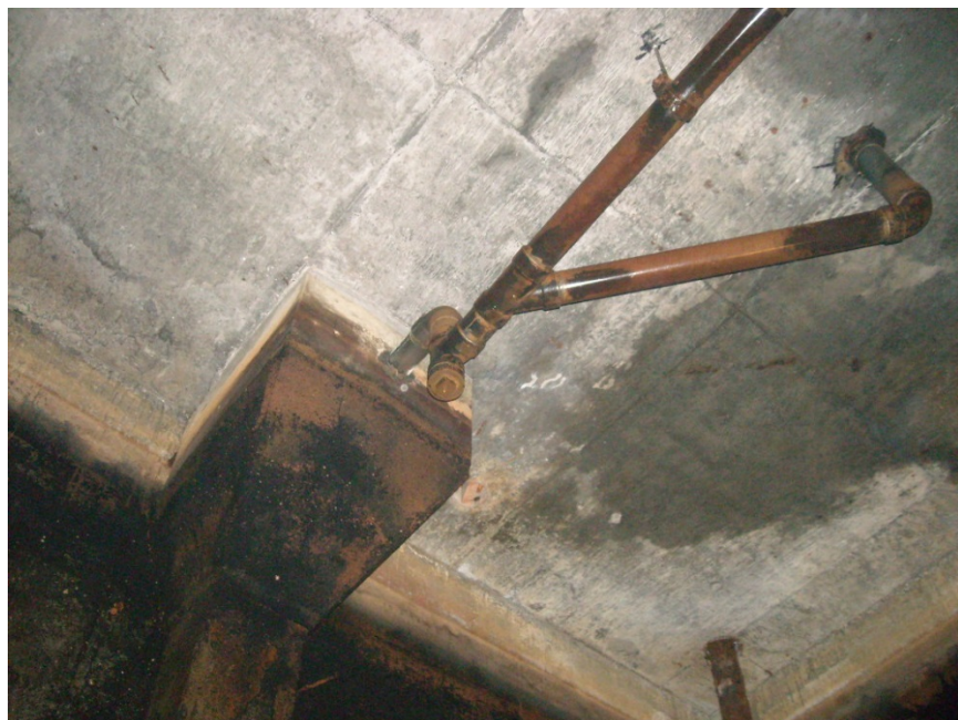
Underside of Main Floor over Clearwell showing Backwash Sump and Floor Drain Lines Photo Supplied by Town Foreman
