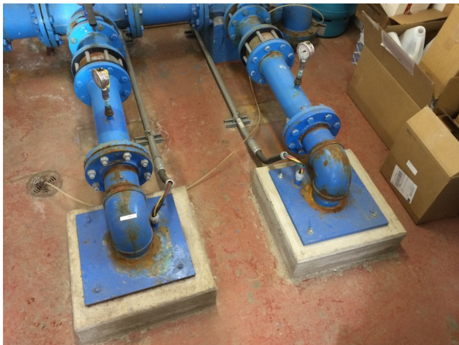
Submersible Distribution Pumps No. 1 and No. 2
