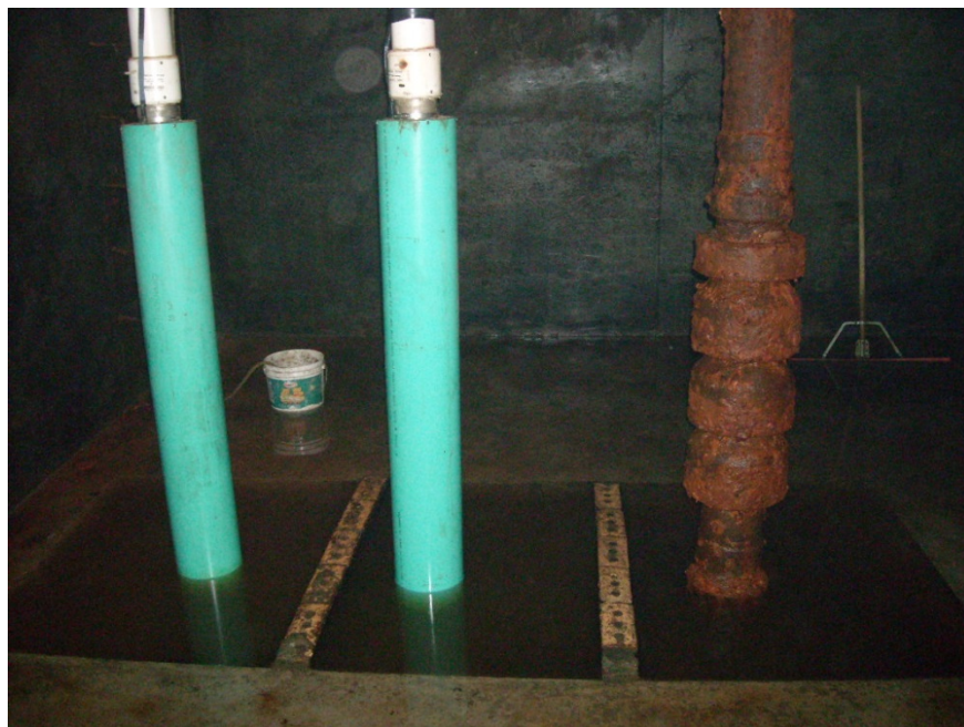
Left to Right: Distribution Pump No. 2, Distribution Pump No. 1 and Standby Pump Photo Supplied by Town Foreman
