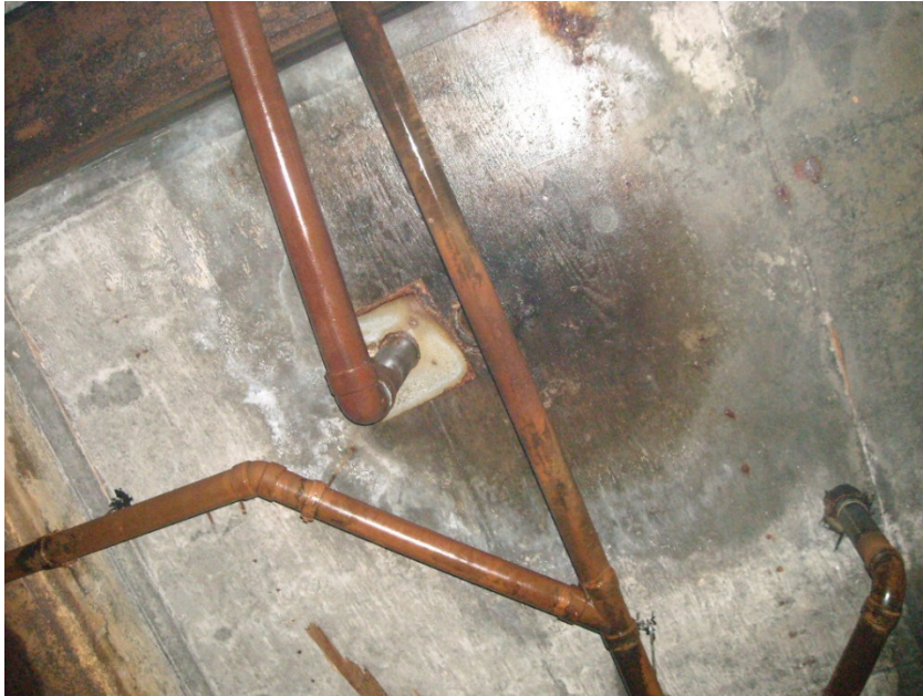
Underside of Main Floor over Clearwell showing Floor Drains Photo Supplied by Town Foreman
