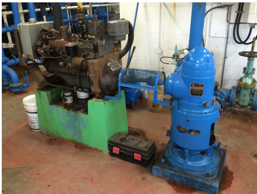
Standby Pumping Unit (Natural Gas Engine, Right Angle Gear Drive and Vertical Turbine Pump)
