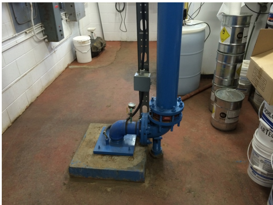
Submersible Distribution Pump No. 3
