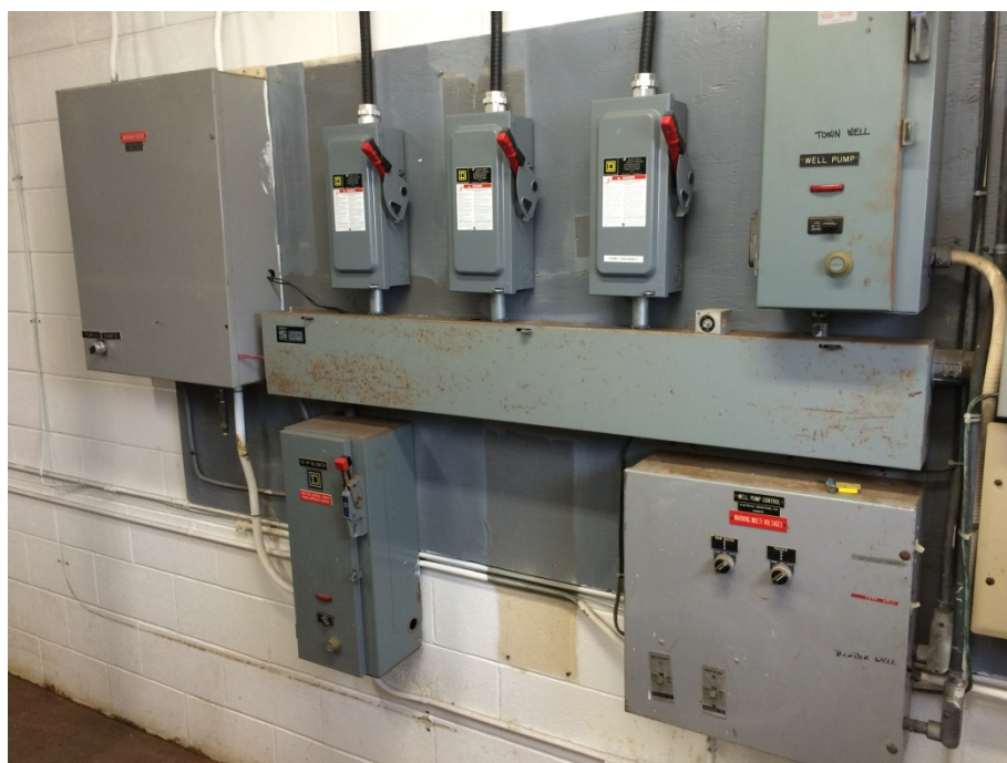
Left Side of Electrical Panel Cluster
