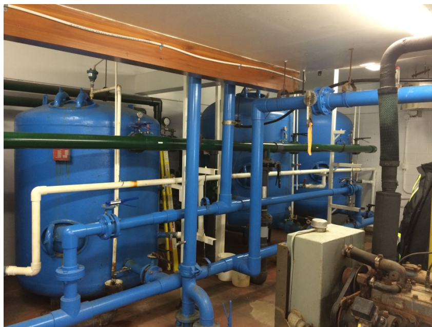
Strasbourg Water Treatment Plant Manganese Greensand Filters
