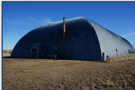
LEAKING ICE ARENA
