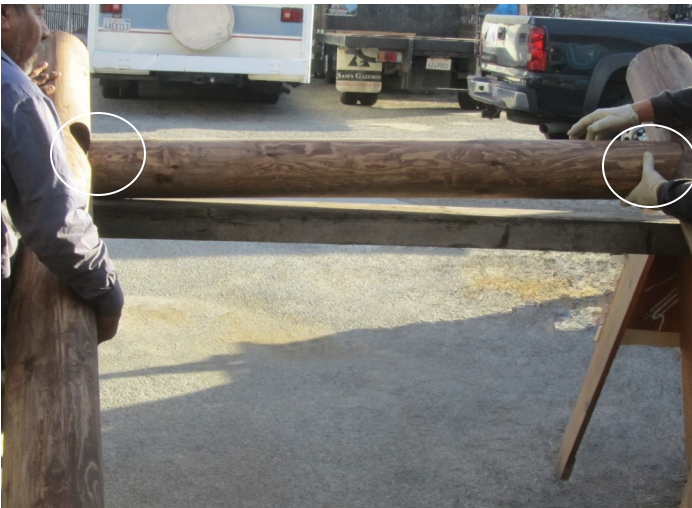
3. Place two Hashira poles with holes inside. Alternatively, you can do it on the ground.
