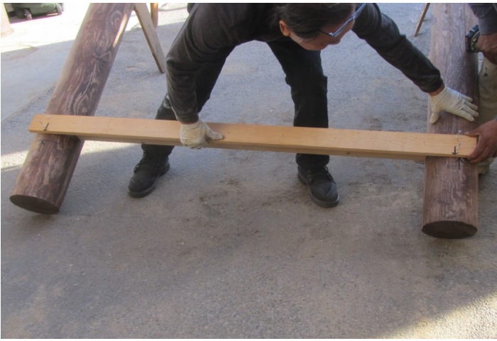
13. Fasten the temporary wood board to the Hashira poles with two screws each.
