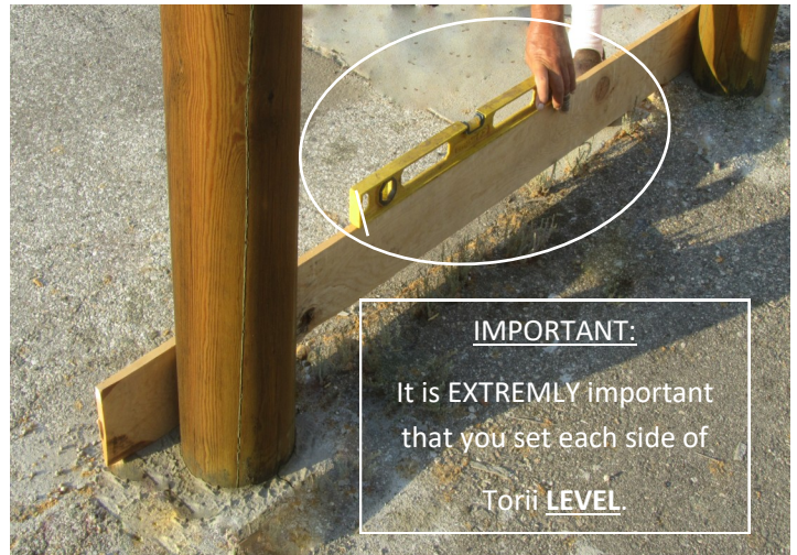
22. Pour mixed concrete into the holes and insert the poles. Check the level and adjust the pole positions if it is not level.
