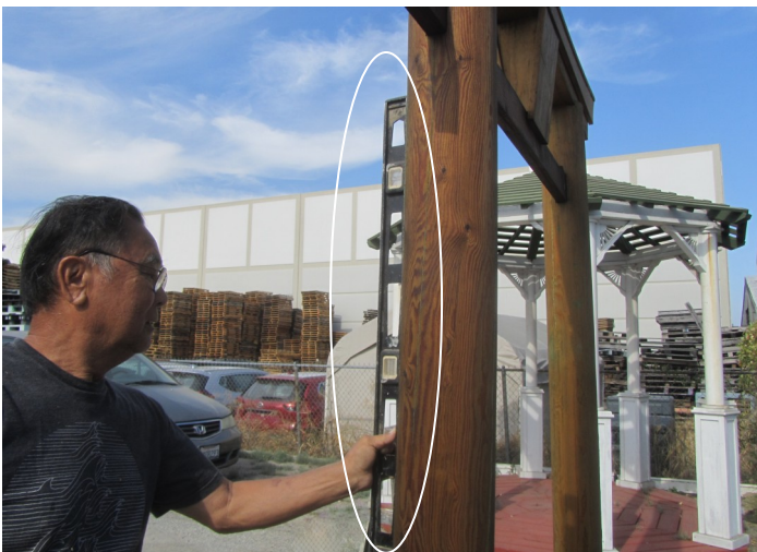
23. Check the level from front or back. Adjust the pole positions if not level.
