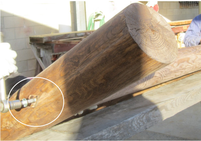
7. Fasten the Nuki and the HASHIRA poles with lag bolts from a side. Leave loose until later.
