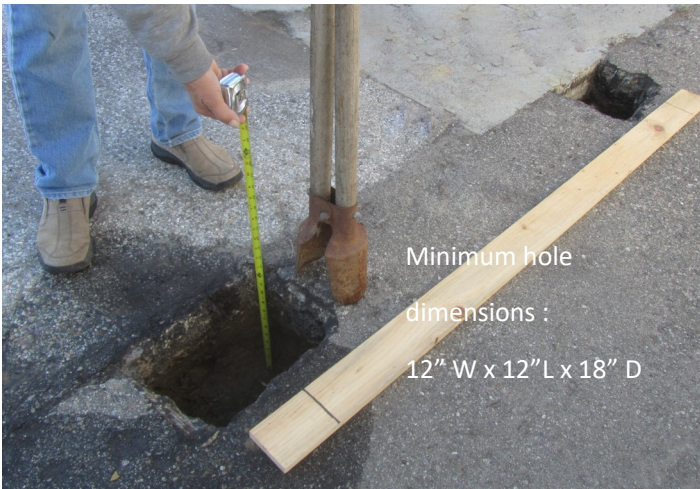
1. Making two holes for Torii poles. Remember that you need to set minimum 6" with cement.(See marks on posts.)
