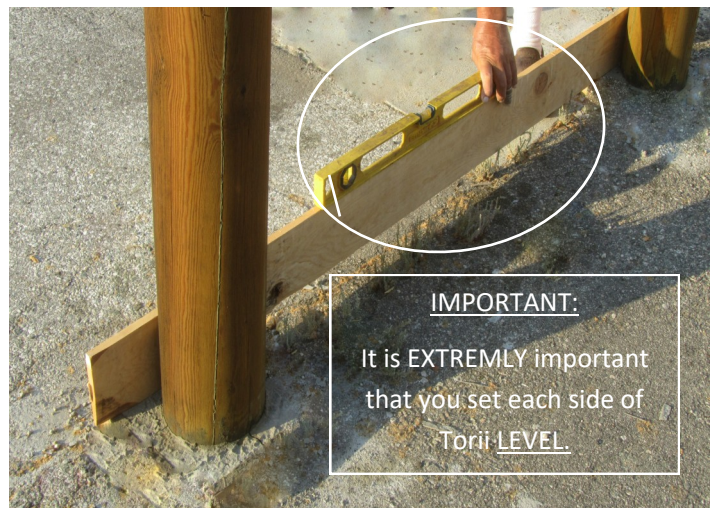
18. Pour mixed concrete into the holes and insert the poles. Check the level and adjust the pole positions if it is not level.
