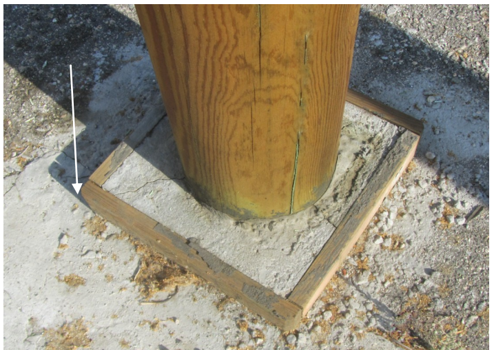
20. Untie the strings to pull down the cement frames, put them at the bottom, and finish the cement work. Remove the extra wood board at the bottom when the cement is cured.
