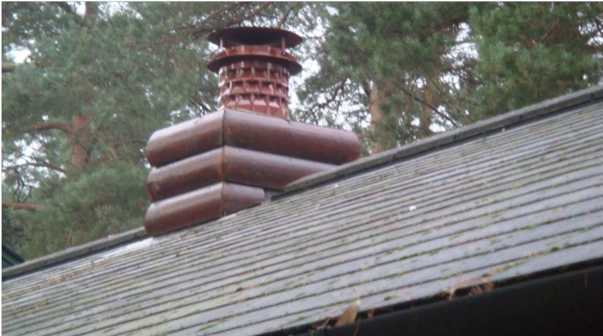
Chimney Sack terminated with 300mm anti-downdraught Windkat cowl
