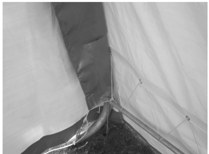
Inside Corner view showing Main Cover and End Panel Door properly laced and secured with turnbuckles.
