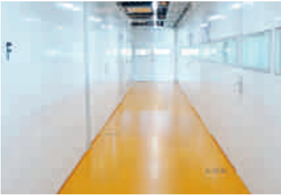
[Fig. 7] Institutes of Pathology and Forensic Medicine, County Hospital, St. Gallen. Metal partition walls can be repositioned and recycled. The reflexion of light contributes to optimal distribution of illumination. Silvia Gmür Reto Gmür Architects (I 1) Bild: © cctp.
