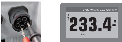
Detecting voltage between L1/L2/L3 and N-wire
