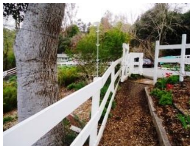
The finished fence: Threaded rods are set into the top of the posts with galvanized wire strung between each post. Wing nuts on each rod hold the wire up. The fence, originally 4 ft. tall, has been converted to 7 foot tall fence but you can build it as high as you like.
