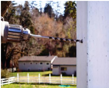
1. Drill 1/2 inch holes through posts to thread the galvanized wire through the post
