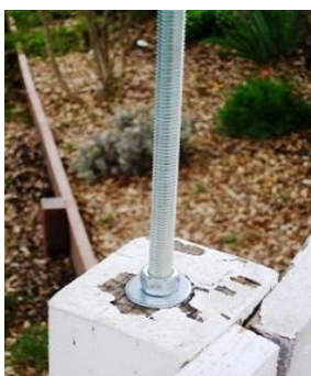
1. A 3 ft. x 1 in. threaded rod is set into the post with a 1/2 in. flat washer and 1/2 inch hex nut secured over the top to hold it.
