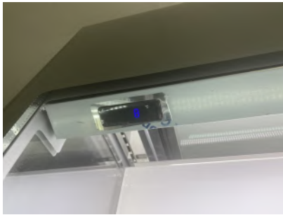
Features a second digital controller in the cabinet space
