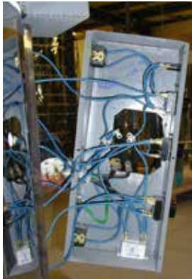
Electrical box without kiln sitter
