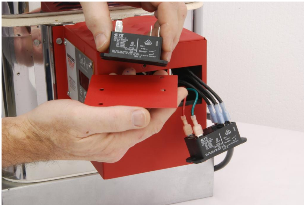
Old relay shown removed from the access plate.
