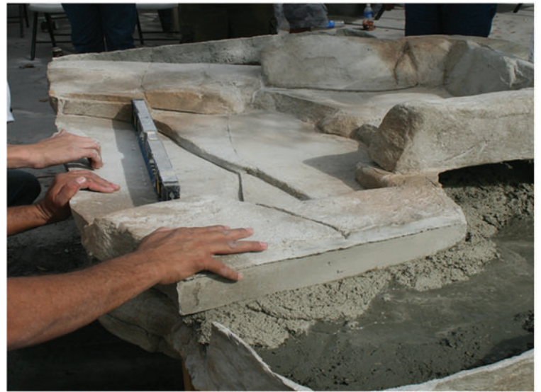
Set grotto top piece #7 in fresh concrete or mortar. It must be level and shape should match the grotto bottom piece. It will drain down when pump is off if set properly.
