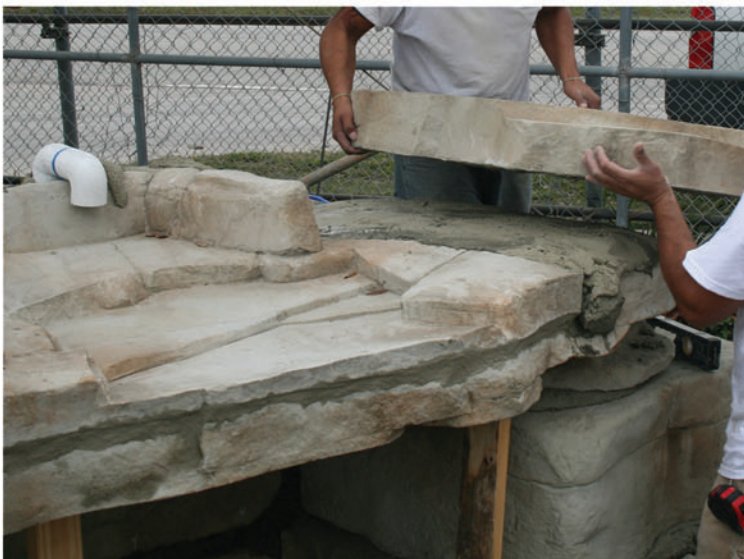
Add 2 inches of concrete fill on each side of grotto top and mortar in top rocks #8 and #9. Add two 90's to 2inch return line to discharge onto grotto top. Set cap rock #10 to hide pipe.
