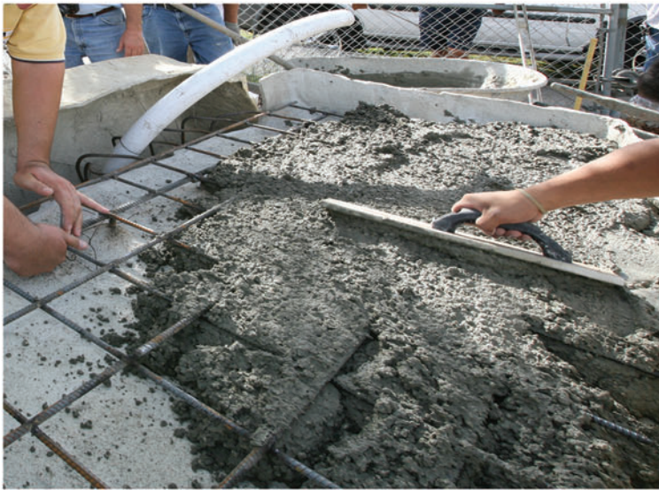
Fill back wall and top with concrete mix, 2000 psi or better. Top should be level. Requires about 1/2 yard of concrete mix.
