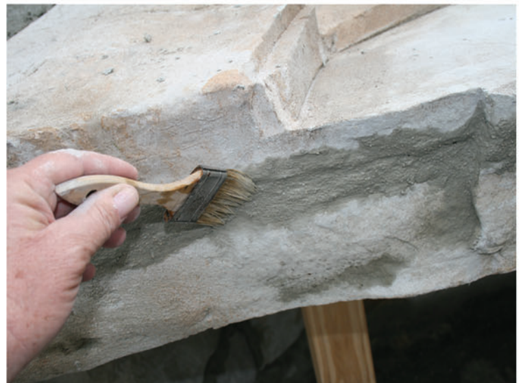
Finish seam between grotto bottom and top. Add accent colors to waterfall pieces. Set small rocks as desired or to divert waterflow. Color touch up after all mortar if dry.
