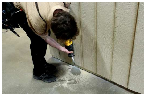
(111) For the bottom of the garage door, where the circular saw can not access, use either the sawzaw or a chisel to cut the bottom.
