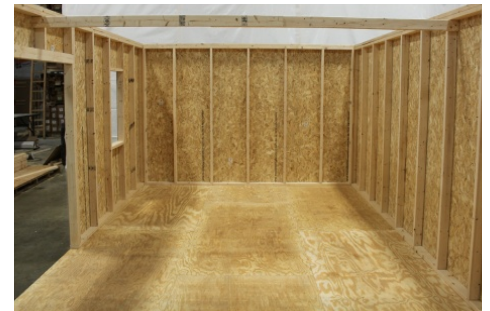
(115) Move the 2x4 wall spacer to just below the top plate, and fasten it on both sides, making sure the walls are pulled in against the 2x4. This will ensure that walls are properly spaced.
