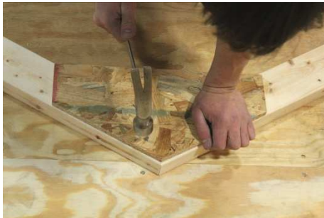
(119) Assemble each rafter by attaching one gusset to each side of the rafters as shown, using a total of ten 2" nails per gusset.
