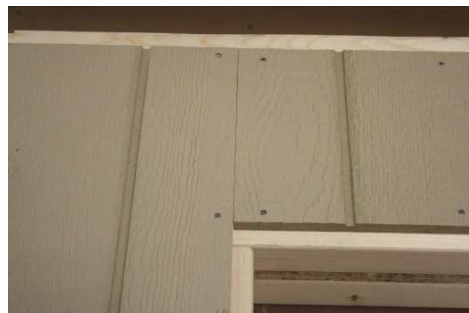
(78) Fasten the siding pieces above the doors, and keep it 3/4" above door header as shown; before nailing.
