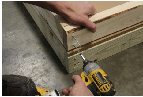
(36) Insert two 3" screws through the pre-drilled holes to attach bottom plate to each wall stud. Make sure bottom plate and wall studs are flush.
