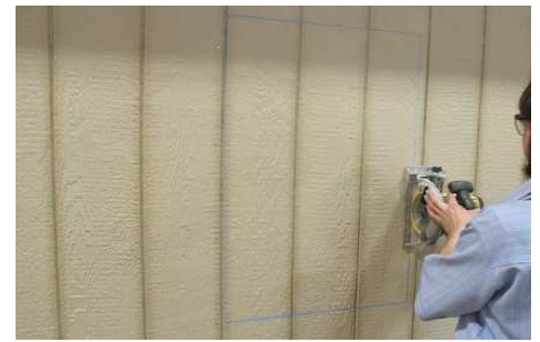
(109) Remove the screws and chalk line, then; set the saw at 1/2", and cut along the lines.
