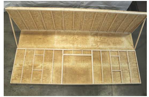
(73) Fasten the rest of the studs, using the same method as the back wall.
