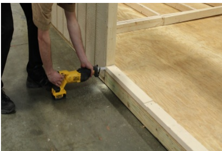
(113) Cut out bottom plate at the double door opening, using a sawzaw.
