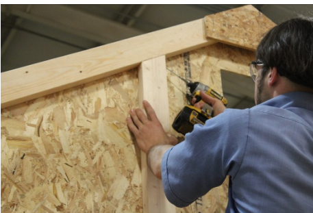
(140) Locate the 4 gable braces then fasten them at the siding splices in the peak, using 3" screws.
