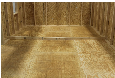
(114) Fasten two 2x4s to each other at the inside to inside width, to be used as a wall spacer, then move to next step.
