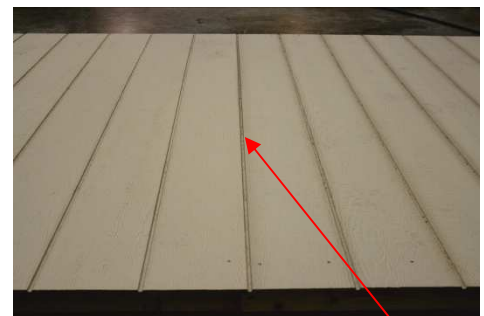
(49) Nail along the splice, making sure the splice is parallel, and looks similar to the other grooves.
