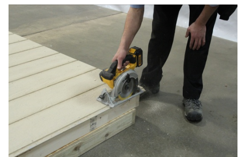
(52) Set the saw to 1/2" and cut along the line so that it is flush with wall frame. Repeat on opposite end.
