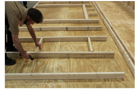
(70) Fasten window studs with dados, to the window blocks, using two 3” screws. Repeat for all the window studs.
