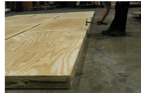
(26) Nail along the front side, making sure flooring is flush with the band board.
