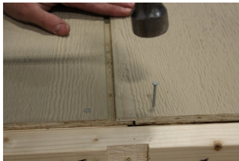
(47) Put the next piece in place, flush with the previous piece, making sure the splice looks similar to the other grooves. Then fasten the corner of the siding to the plate.
