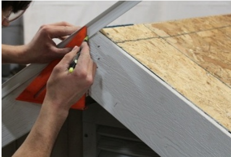
(209) Make a mark on the drip edge, parallel with the gable splice.
