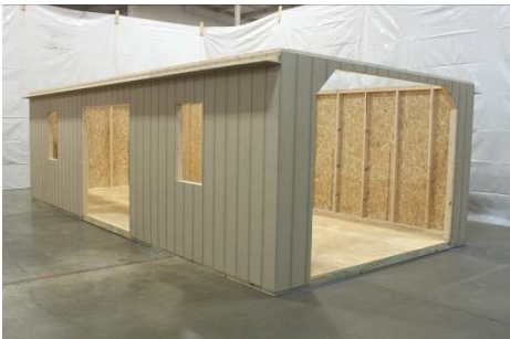
(110) Repeat for the other window, and also the garage door, using the same method.
