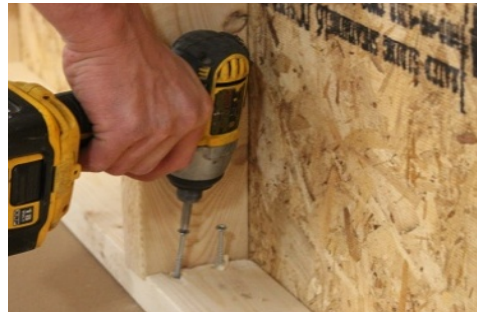
(63) Repeat for the rest of the wall, again; making sure wall is in against the floor frame.
