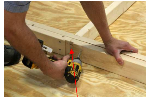
(39) Before fastening the double top wall plate, ensure that dado grooves align with wall studs, and are faced outward.
