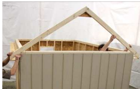
(120) Begin with end rafter keeping single gusset facing to interior of shed as shown.
