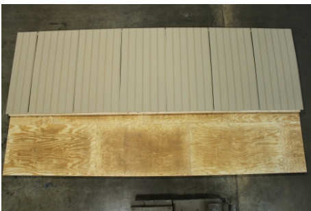
(41) Lay out siding as shown here, with the overlap towards the left.
