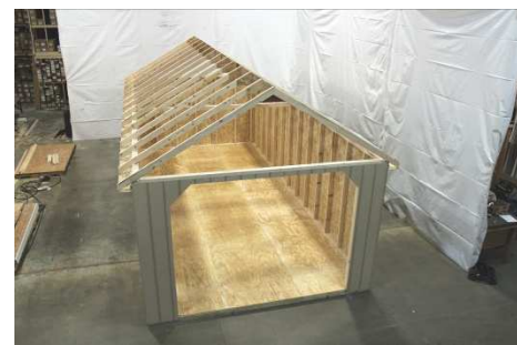
(124) Install the rest of the rafters, 24" on center, or in every dado groove on the top plate. Repeat, till all rafters are installed.
