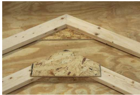
(117) Lay out the rafter pieces and the gussets. Note: Two rafters will be assembled using only one rafter gusset, the remaining rafters will be assembled using two rafter gussets.
