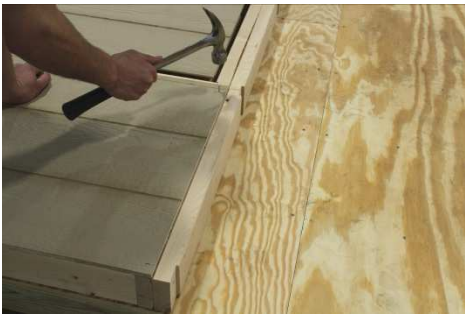
(44) Nail along the top, after making sure the siding is flush with the center of the double top plate as shown. Use an 8" to 12" nail spacing.
