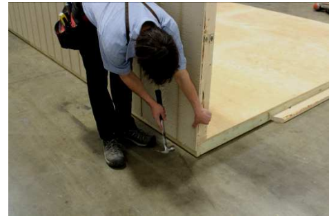
(64) Attach bottom edge of siding to floor, using an 8” to 12” nail spacing. Do not leave the back wall standing alone, without firmly bracing it.
