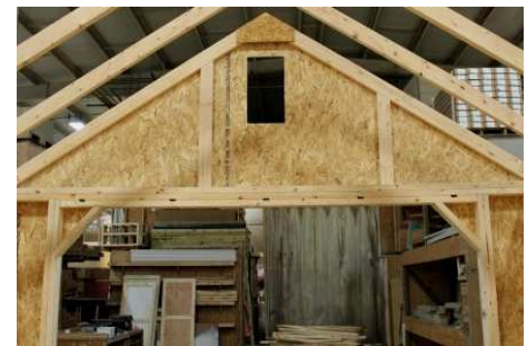
(142) Fasten the other gable brace on this gable, then repeat for opposite gable. Next, fasten the siding splices to the gable braces on the outside.
