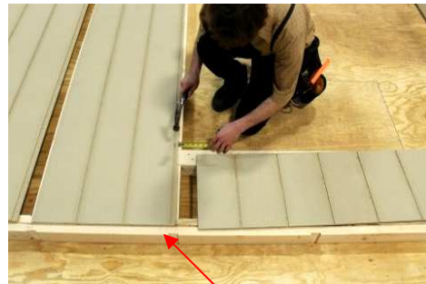
(75) Starting with the piece beside the door, place the siding even with the center of the double top plate, then make sure siding has 3/4" reveal along edge of door frame, before nailing.
