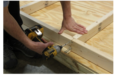
(37) Repeat the process for the rest of the wall studs; but use four 3" screws as shown, for any splice.
