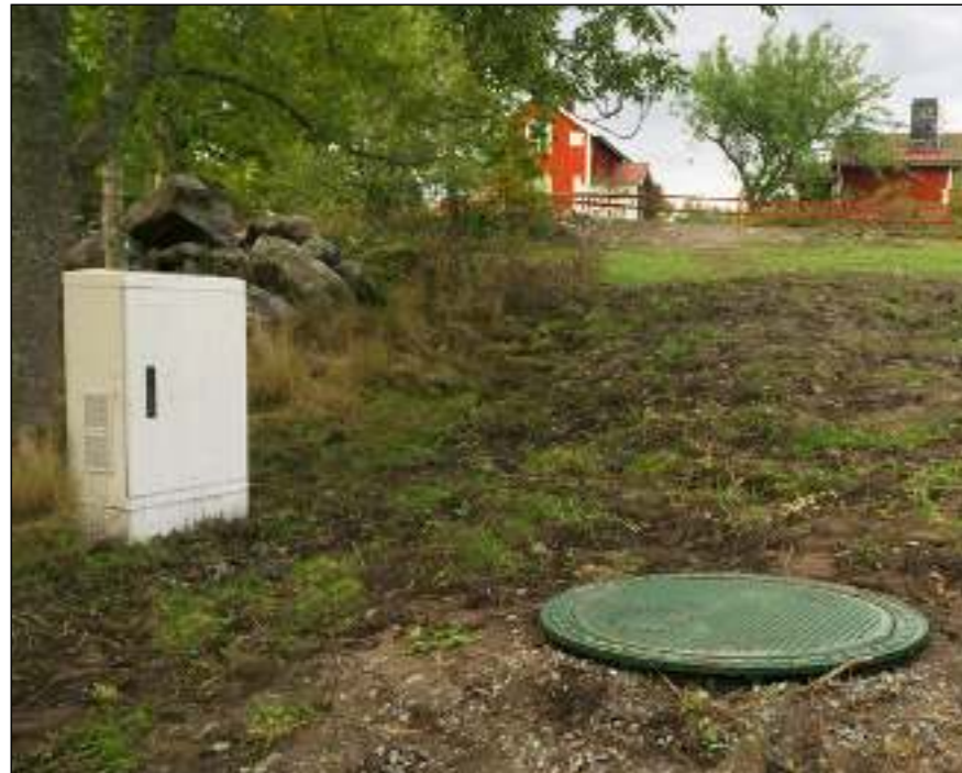
The image shows the External plastic cabinet L with LED warning light for 20 inhabitants
