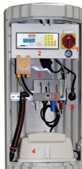
Open external switch cabinet
