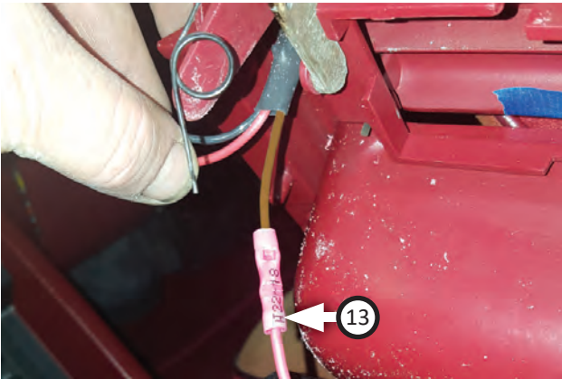
17. Use splice (13) to connect solenoid power wire (that was routed through firewall to center console) to brown wire on lit momentary switch.
