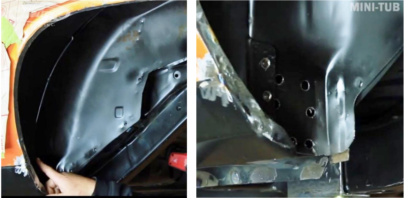
Figure 12 - Drill Wheel Tub Spot Welds
