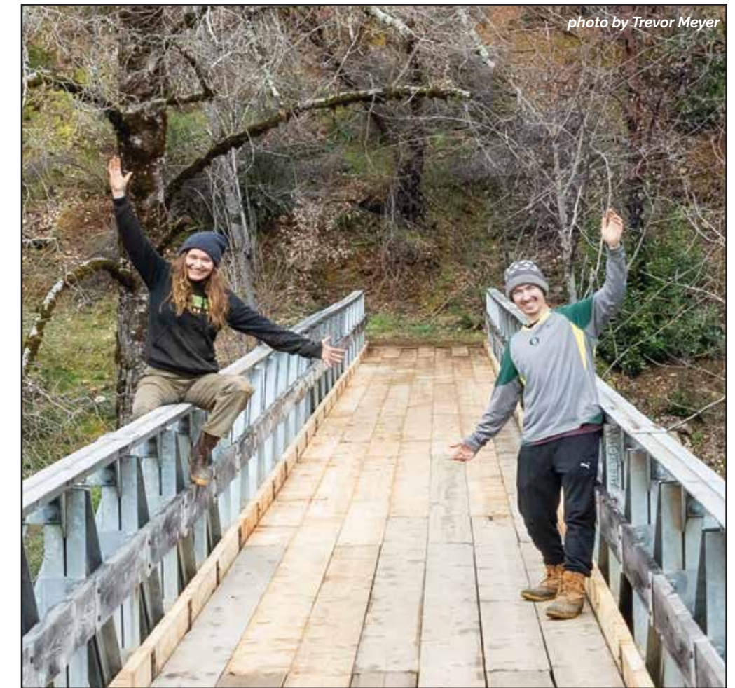
ABOVE: Program directors Karly White and Trevor Meyer celebrate the completion of the Briggs Creek Bridge, located at the trailhead for the the Illinois River Trail.
