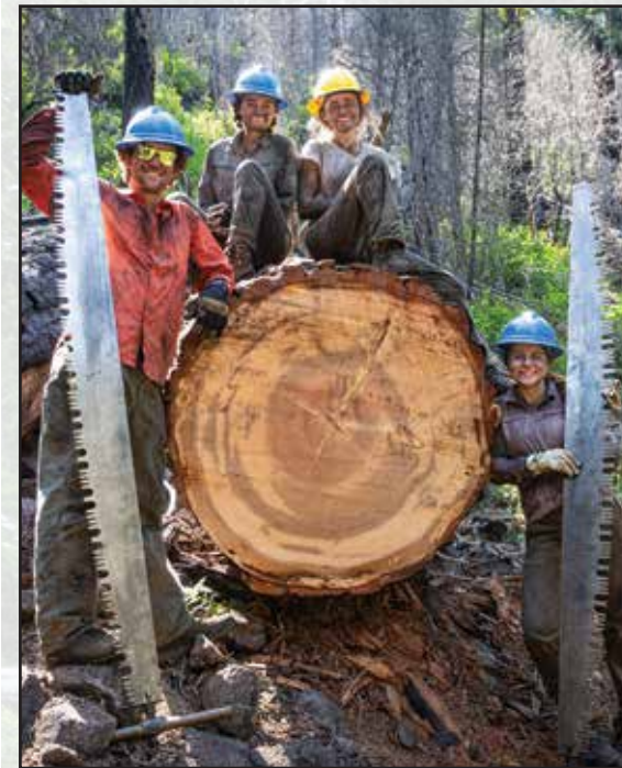
Above: Our 2021 Wilderness Corps spent several days clearing massive logs along the Clear Creek National Recreation Trail. | photo by: Trevor Meyer
