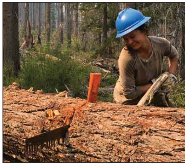
Above: 2021 Intern Anna Slager using the single crosscut saw while working on the Middle Fork Trail #978, Sky Lakes Wilderness. | photo by: Owen Brodie
