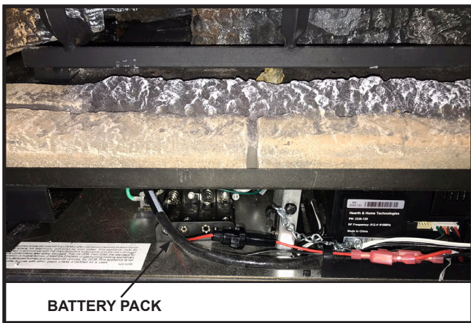
Figure 3.8 Battery Pack Installed
