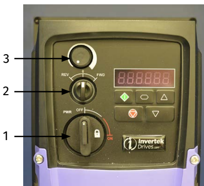
Fig. 8a Pump operation switches
