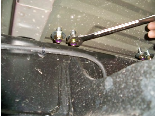
(Fig. 13) Install washers and nylon locknuts on the exposed bracket studs underneath the bed. Tighten the locknuts to 40 ft. lbs.
