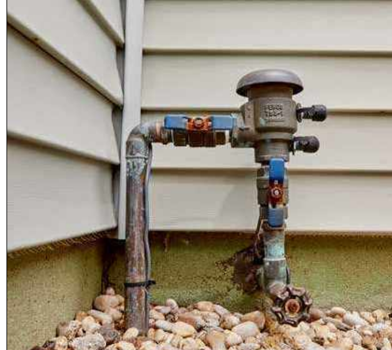
SPRINKLER SYSTEM BACKFLOW ASSEMBLY
