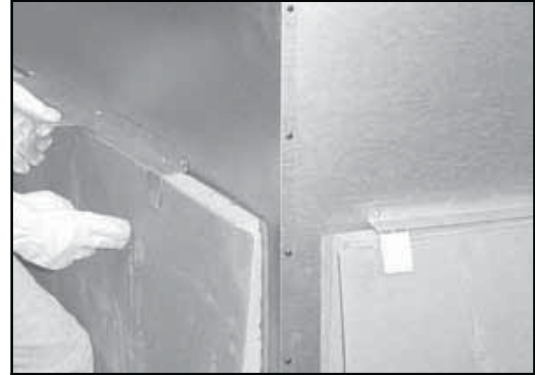
Figure 7.1 Unpacking Back Refractory
