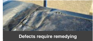
Defects require remedying
