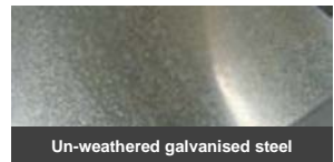
Un-weathered galvanised steel
