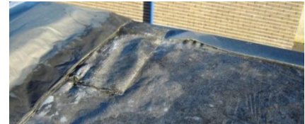
Defects require remedying
