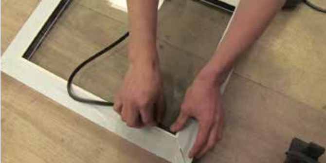
7 Take the wedge gasket and starting at the corner push it in between the glazing and aluminium vent.
