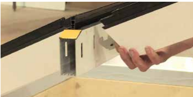
5 Where there is no hidden tie bar position the bracket into the slot on the ridge and fix rafter with screw.
