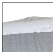
WHITE WATERPROOF ROOF MATERIAL
