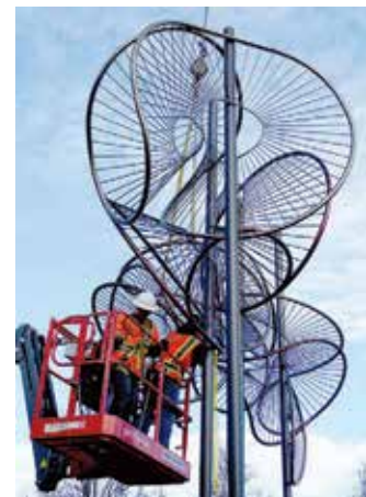
Workers install Susan Zoccola's, "Threshold" in the gateway site on Groundhog Day.
