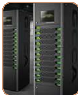
UPS uninterruptible power supply
