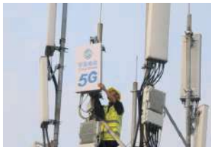
base station back up
