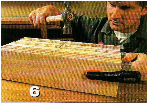
6 All staples should protrude out of the louver about 1/4 in. Tap down high staples with a tack hammer.
