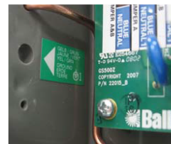
Ground in System Enclosure
