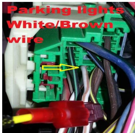
Figure 2. Parking light wire
