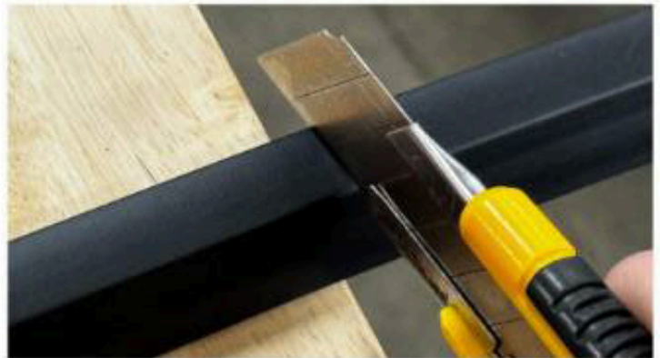
28. Heating the wire hider may be required due to memory. Measure the distance between lights and cut wire hider with sharp razor. Clean surface and tape to rail. Repeat for the other side.
